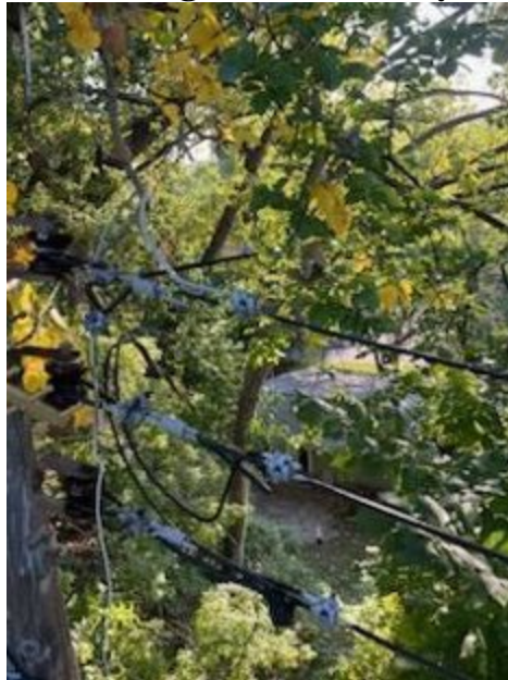
Figure J-1: Vegetation Causing Power Quality Issues Detected by DI
